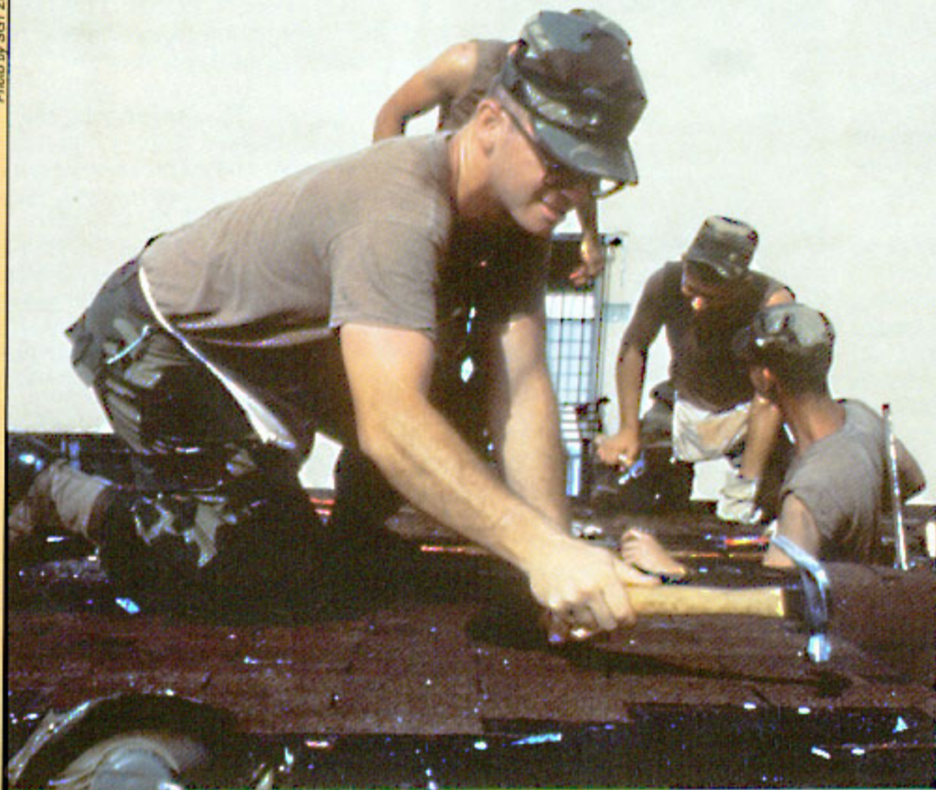
SGT Scott Anderson, 10th Mountain Div (L), Ft. Drum, NY, hammers shingles on a roof top at a local resident's home in Homestead AFB, FL as part of the Hurricane Andrew relief mission.
